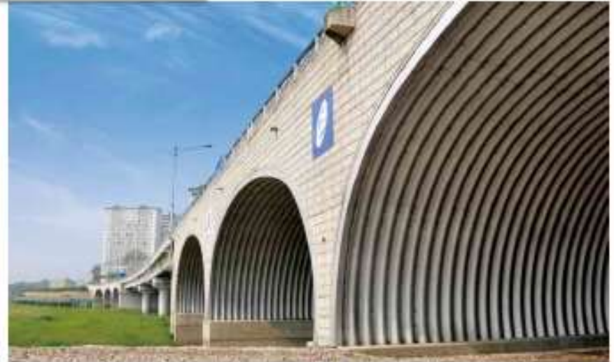
Ranong-Silong Gorge Bridge (Gesungdo/Construction Headquarters/2009) | Type : Low profile arch / Span : 17.0m / Rise : 6.7m / Length : 20.0m
