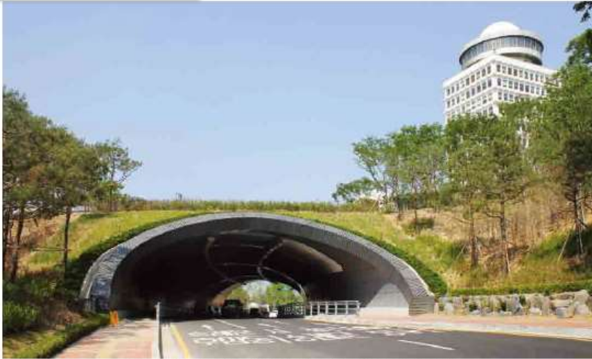
Namsan Haebyeon Eco-tunnel (Good/2012) | Type : Low profile arch / Span : 18m / Rise : 5.5m / Length : 70m
